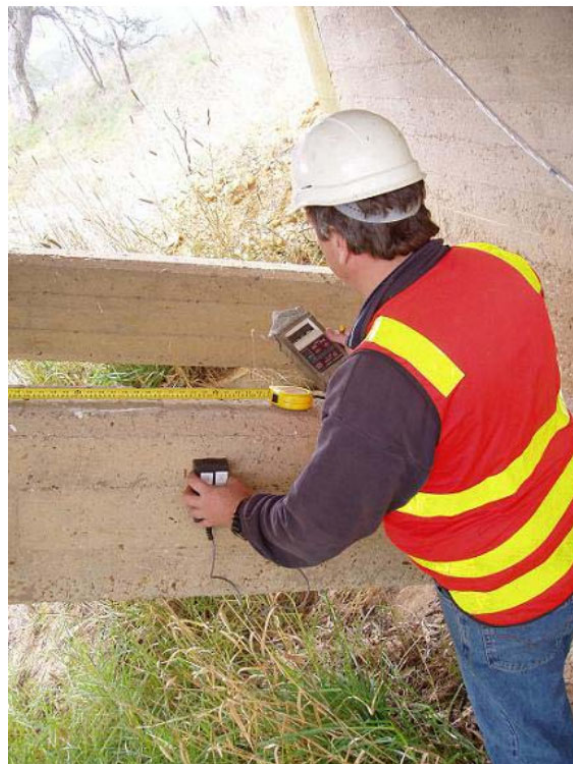
Mod Shock testing to check the integrity of bridge foundation and pile system
