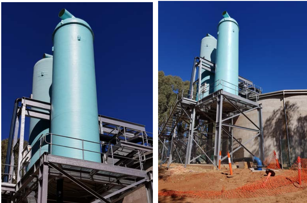
Second Aerator Tower.
